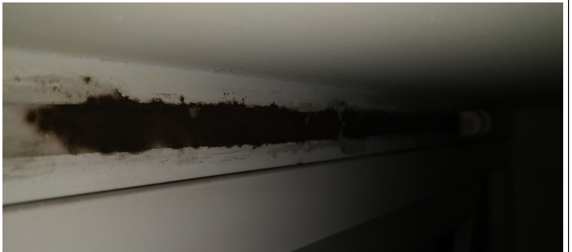
47 White framed double glazed window, 1 opening with white handles Air vents missing and filled in to RHS, tape marks and scuffs around frame, mildew marks to LL sealant
